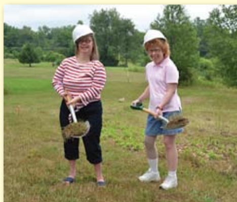
Adrienne Motz and Amy Russell take out the first shovels of dirt for the construction of the new Chosen Vision DeWitt home.
